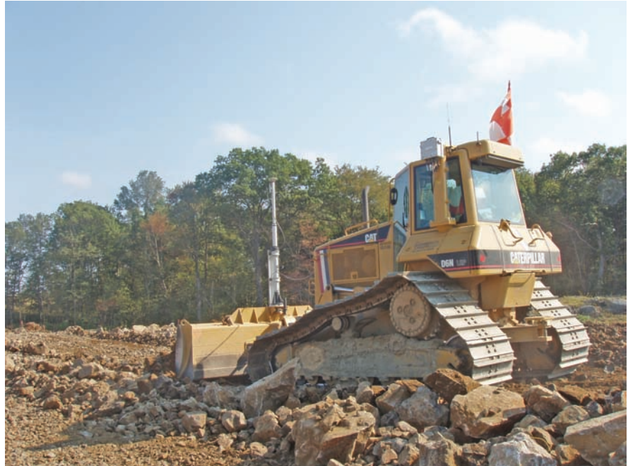
Also equipped with a Leica GPS system is this CAT D6N. Note the red and white checkered flag required when working near an active runway.
