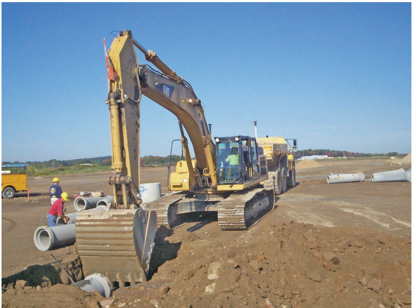
A CAT 345 excavator equipped with a Leica GPS system digs trench for a storm pipe at the Beverly, Mass., airport.
