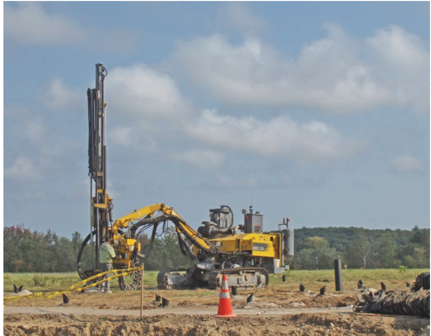
Maine Drilling & Blasting employs an Atlas Copco ROC D3 drill to bore holes for the blasting of some 5,000 cubic yards of rock.
