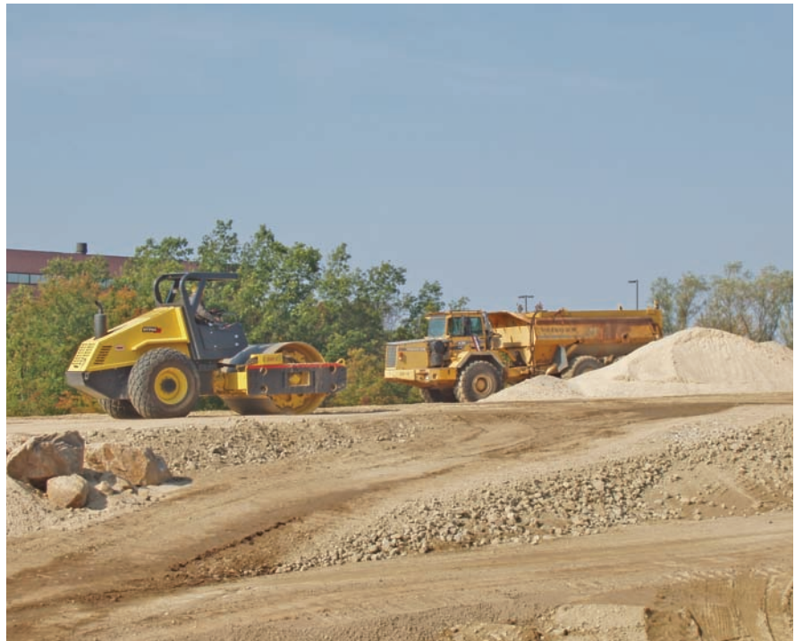
A Dynapac 840C vibratory steel roller compacts gravel fill while a Volvo A35 off-highway truck delivers more gravel.
