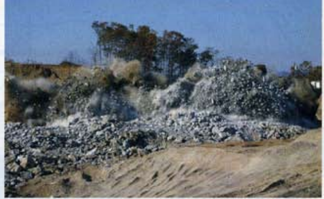
Shooting three times a day on average, blaster filled boreholes with up to 4,000 pounds of explosives per shot.
