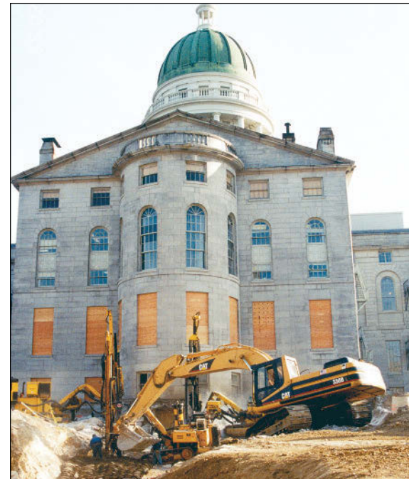
Photo courtesy of Maine Drilling & Blasting In 2000, a $32 million renovation of Maine's historic State House and State Office Building, located in Augusta, called for the replacement of a 150-ft. (45.7 m) walking tunnel. The Maine Drilling & Blasting Company was called in to remove approximately 3,000 cu. yds. (2,294 cu m) of rock from an area directly below the 110 year-old landmark.
