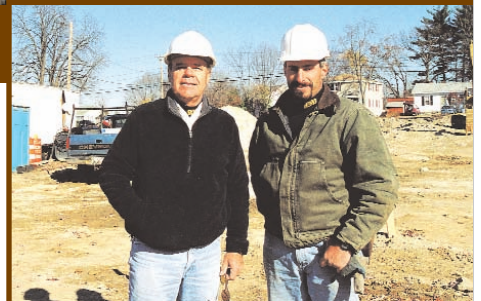
John Swiniarski, owner, and Tim Orio, job superintendent, of Jakon Development Inc., discuss progress of site work.
