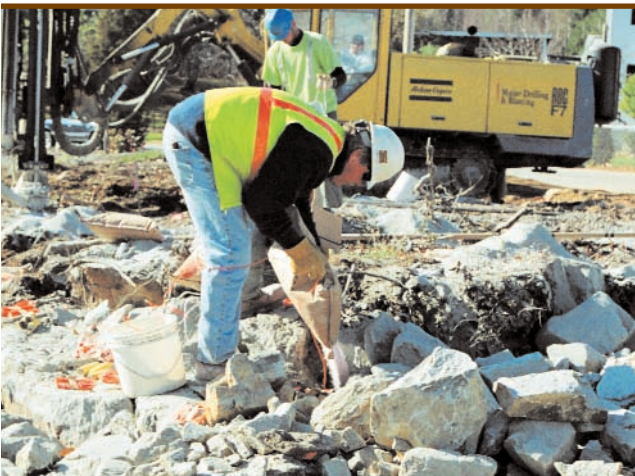
Maine Drilling & Blasting crew loads ANFO explosives into holes bored by Atlas Copco drill at rocky site for Jakon Development Inc. subdivision in Dracut, Mass.
