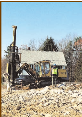
Subcontractor Maine Drilling & Blasting's Atlas Copco ROC F7 drills holes on exceptionally rocky site.
