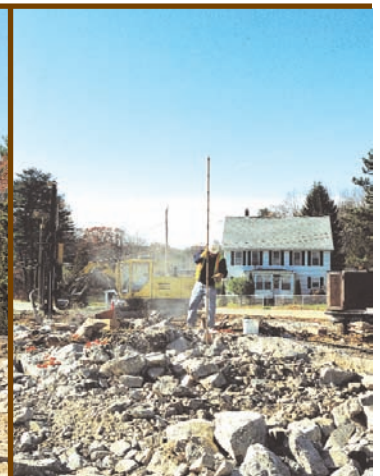
Blaster checks depth of ANFO explosives in one of the drilled holes.
