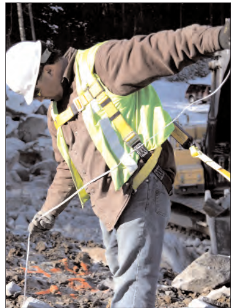
Mike Lupone loads charges in a hole on the future site of a Rochester, New Hampshire Walmart.
