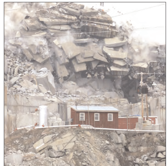
Removing waste rock at Rock of Ages in Barre, VT; MD&B have executed over one million blasts in their 40 years.
